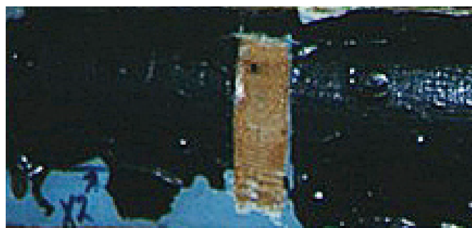
FIGURE 5.17 Damage to painted surface caused by paint chip sampling.
