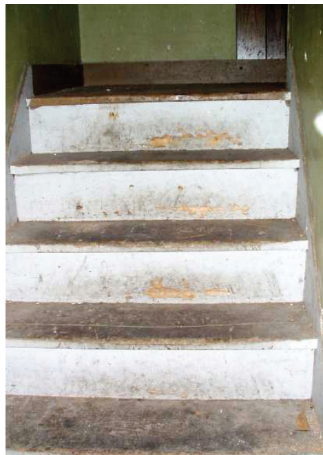
FIGURE 5.6a Friction hazard on stairs pre-treatment.
