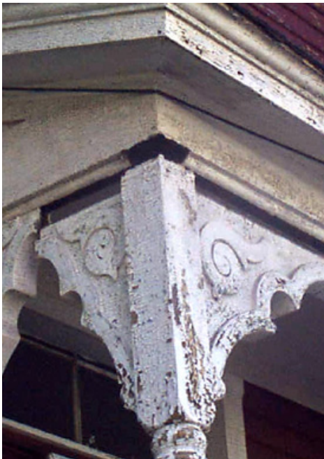
FIGURE 1.2 Deteriorated residential paint on house trim.
