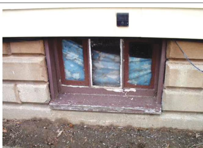
FIGURE 6.3 An area of bare soil beneath a window with deteriorated paint.
