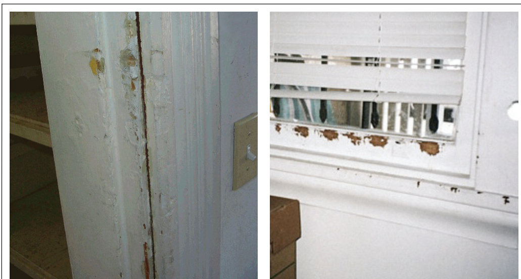
FIGURE 11.4 Examples of impact surfaces (left) and chewable surfaces (right). The window sash has large teeth marks.
