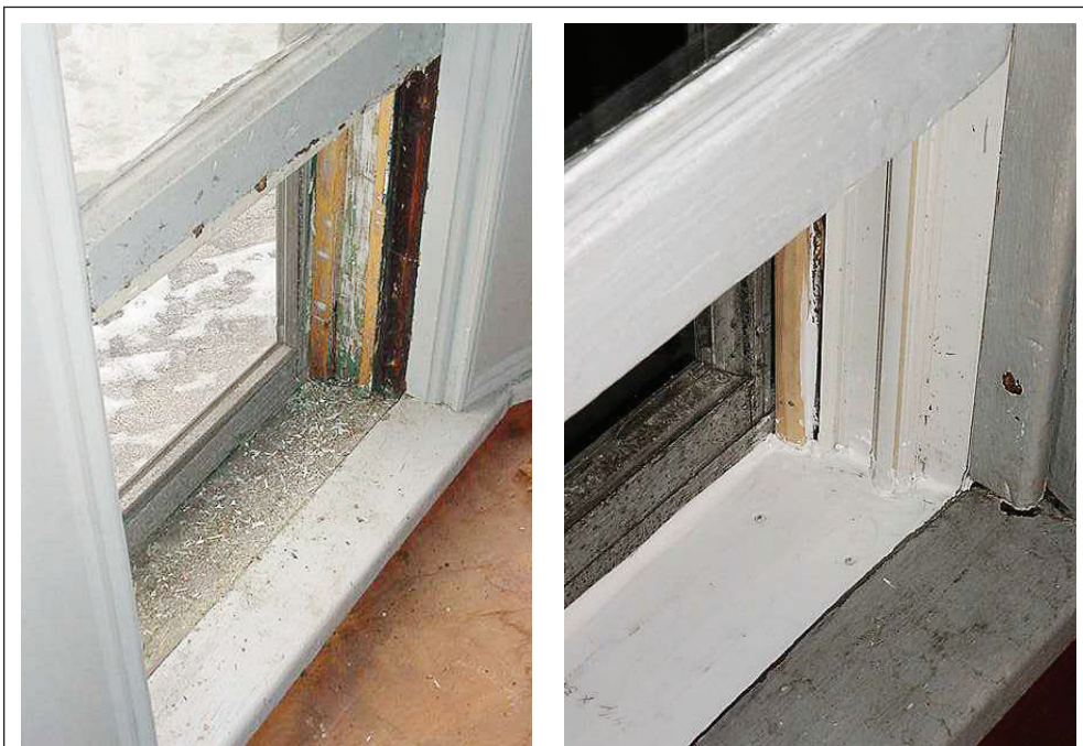
FIGURE 11.3 Window before and after friction treatment.
