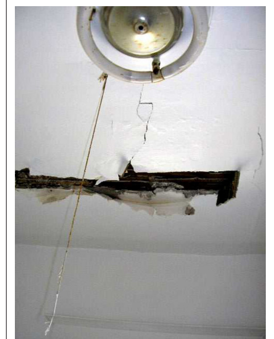
FIGURE 8.4 Example of structural deficiency needing repair prior to work.
