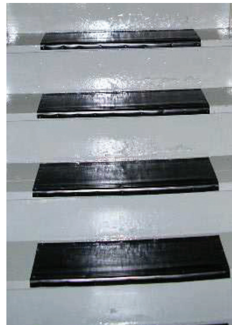
FIGURE 5.6b Friction hazard on stairs post-treatment.
