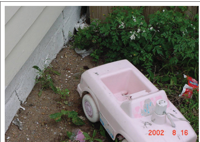
FIGURE 5.9 Soil lead hazard at dripline
