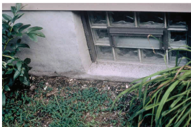
FIGURE 15.2 Visible paint chips and debris in the soil.
